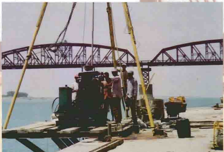
Exploratory Bore Holes by Rotary Drill Rig on River at Paksey Bridge Construction Project.
