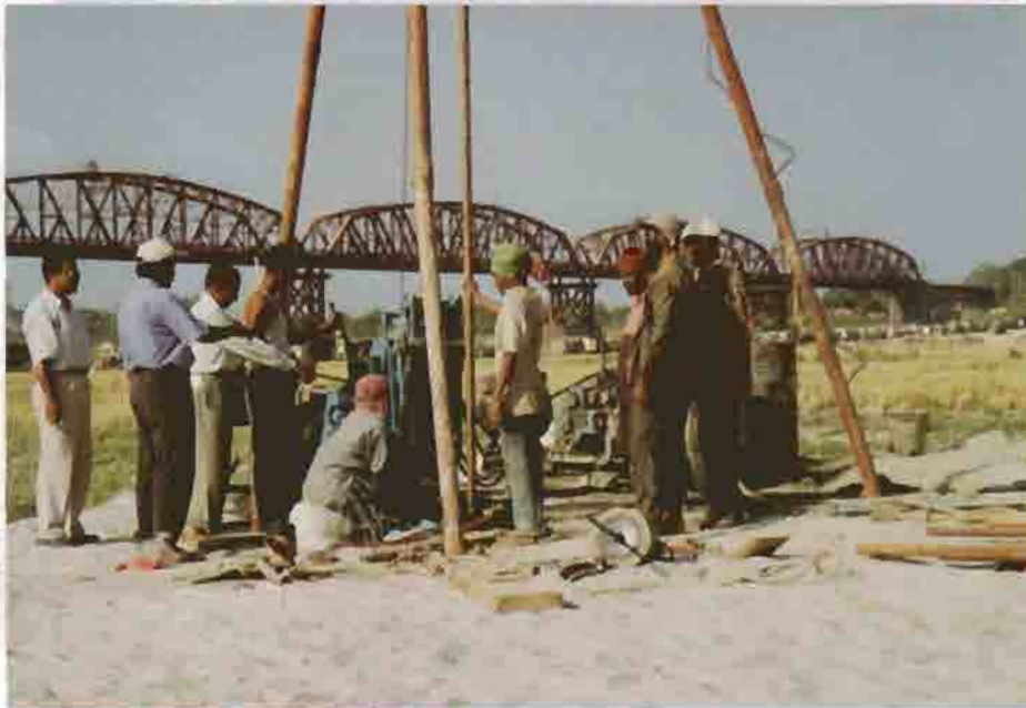
Exploratory Bore Holes by use of Rotary Drill Rig on Land at Paksey Bridge Construction Project.
