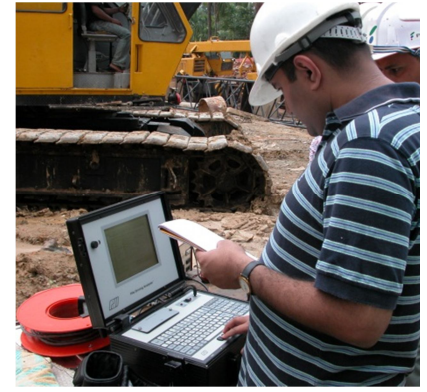
Pile Driving Analyzer (PDA)
